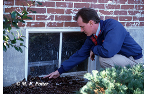
Fig. 5: Do not allow mulch to contact wood siding, doors and windows.
