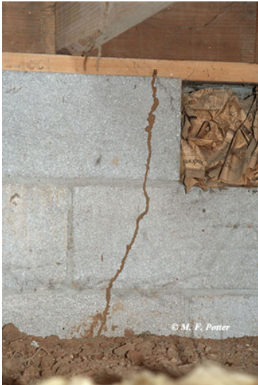
Fig. 6: Telltale signs of termites: mud tunnels
