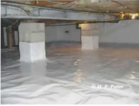
Fig. 3: Moisture in crawl spaces can be reduced by installing plastic sheeting.
