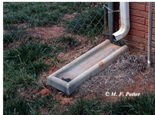
Fig. 2: Divert water away from foundations. Downspout splash blocks are helpful, but this one is facing in the wrong direction.
