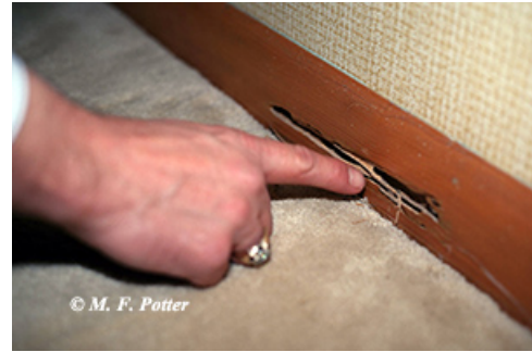
Fig. 8: Telltale signs of termites: damaged wood with soil in the galleries.
