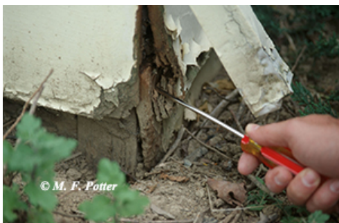
Fig. 1: Wood-to-ground contact aids entry into buildings.
