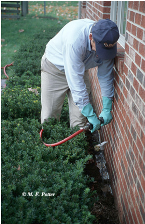
Fig. 3: Termites can also be controlled by treating the soil with a liquid termiticide.
