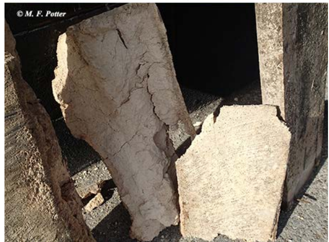
Beetle damage in a rickhouse. It took many years to reach this point.
