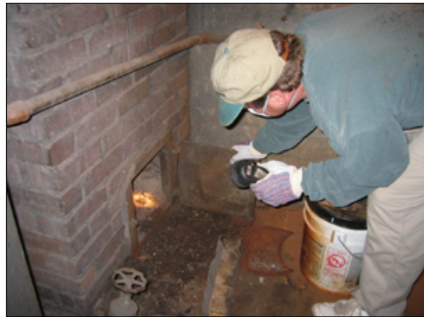
Inspections in secluded areas require a bright flashlight (work gloves are also recommended) (M. Potter, Univ. Kentucky)
