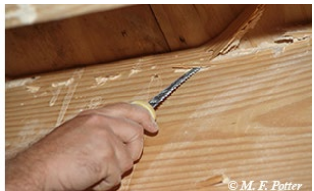
Fresh powder sifting from recent emergence holes. Damage may be evident just below the wood surface.
