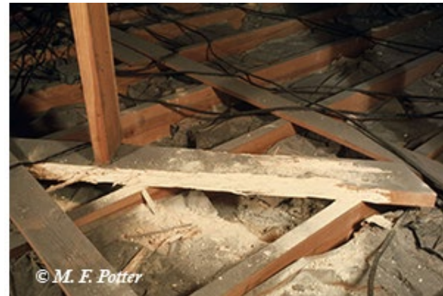
Significant damage can occur in humid, poorly ventilated crawlspaces and attics.
