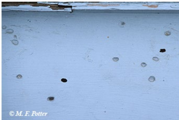
Old house borer emergence holes. Some of the holes in the exterior siding have been sealed and painted over.
