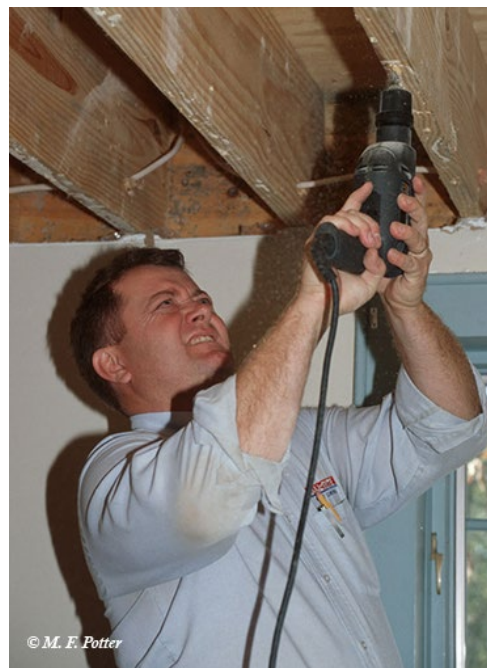
Insecticides can also be applied by drilling and injecting directly into infested wood.
